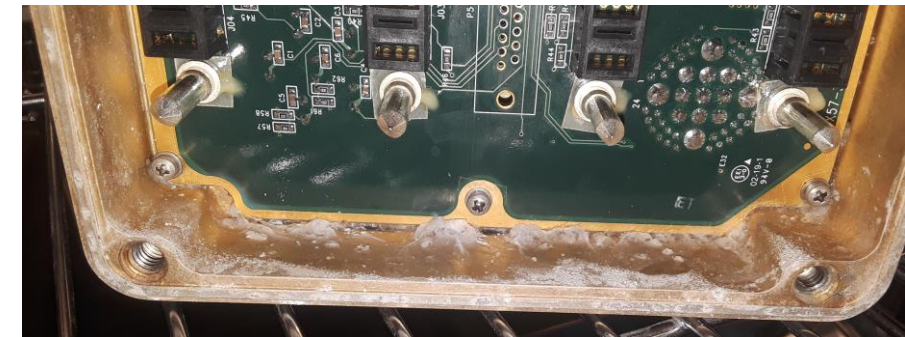
Corrosion Intrusion Due to Primary Seal Failure
